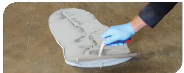
A small amount of moisture on a trowel will allow the surface to be finished smoothly. Re-wet tool frequently to prevent dragging.
